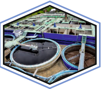
Water Treatment Plant Hafeshwer P6
